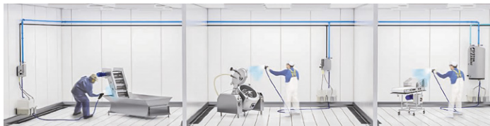
Figure 4: Two remote satellite (left and center) and one medium-pressure (right) stations. All stations: a booster station and an integrated satellite POU
