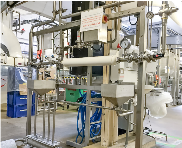
Figure 7: Capsule Filter Horizontal Installation at POU
