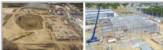
Yauco | Puerto Rico: Start of building additional capacity for filters and bags
