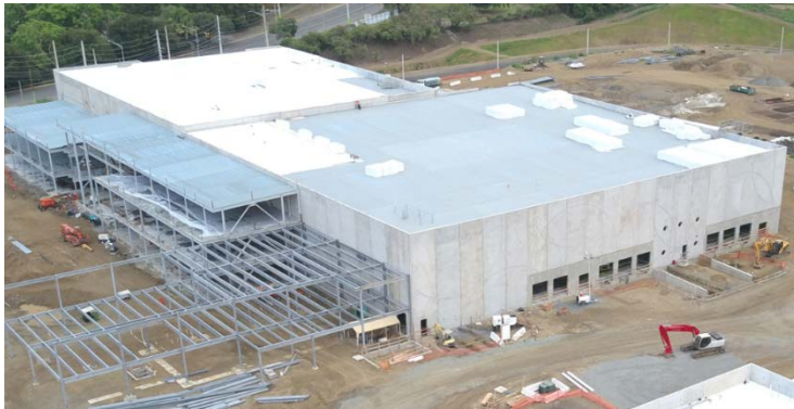
Yauco, Puerto Rico Doubling of fluid management and filter capacities
